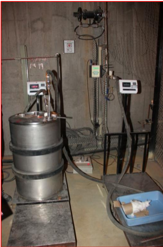
D 2 O addition area in KAPP-3
