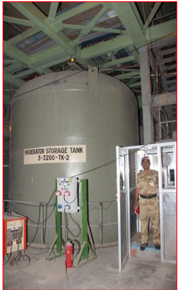
CISF Security provided near Moderator Storage tank (3-3200-TK-2)
