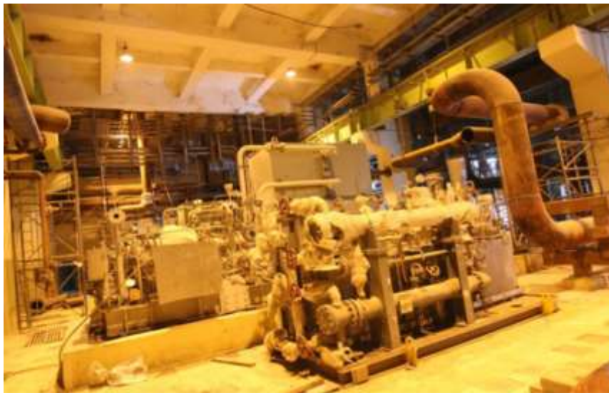
BOILER FEED PUMP UNIT
